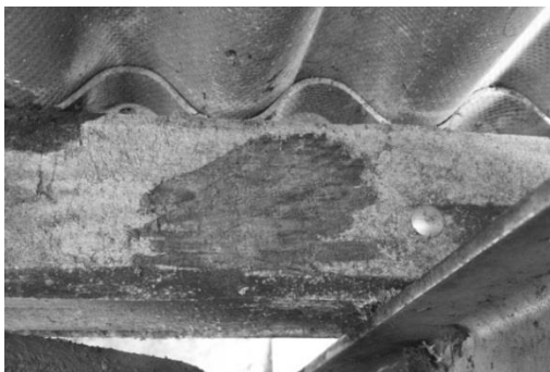
Figure 2. Wooden beams exposed to fungi.
