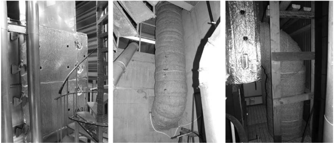
Fig 6. Example of grain dryer insulation.
