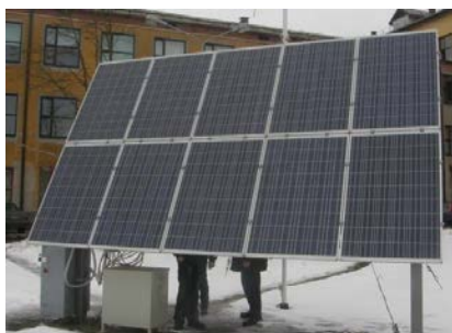
Figure 2. Two kilowatts PV array of 10 Kioto KPV 195 PE modules.
