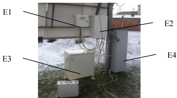
Figure 4. Placement of enclosures of electrical equipment: E1 – solar charge controller; E2 – inverter; E3 – VRLA batteries; E4 – dedicated wind turbine charge controller.
