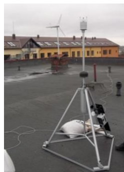
Figure 3. Vaisala weather station MAWS201 and 300 W wind generator.
