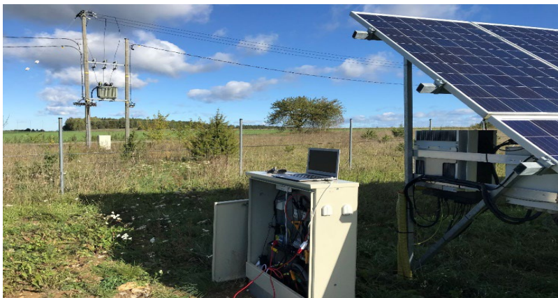
Figure 3. Solar Power Plant point of common coupling (PCC) with a 10 / 0.4 kV substation in the background.
