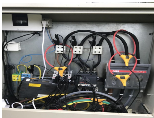
Figure 4. Main switchboard and PQ measurements.
