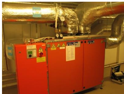
Figure 3. The heat exchanger Menerga 191101.
