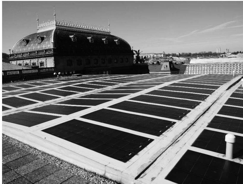
Figure 3. PV power plant on the National Theatre roofs (Service Building).
