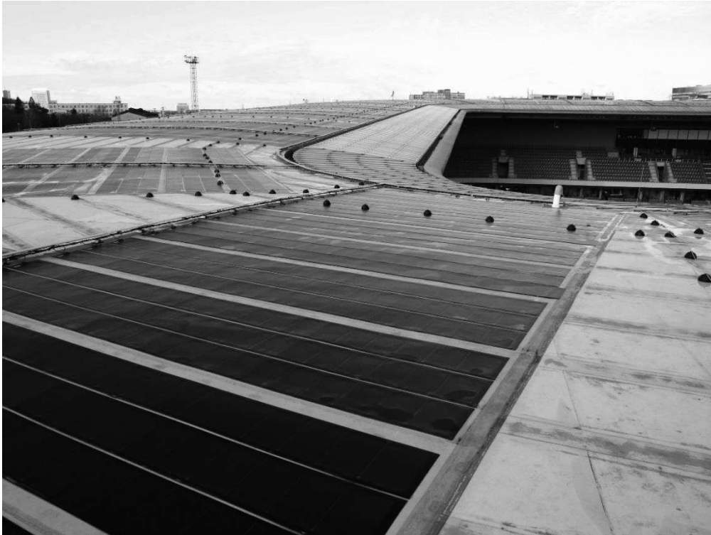
Figure 9. PV power plant on the roof of the SK Slavia football club, Prague.
