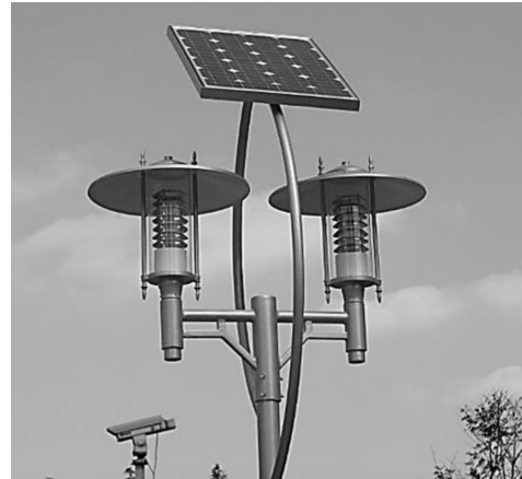
Figure 1. Autonomous PV system for street illumination in Shanghai.
