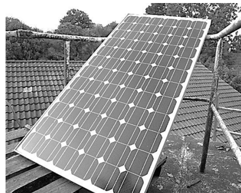
Figure 2. Outer part of the PV system - PV panel.
