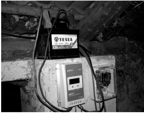
Figure 3. Lead acid accumulator with charge regulator with MPPT.
