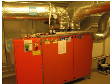
Figure 3. The heat exchanger Menerga 191101.
