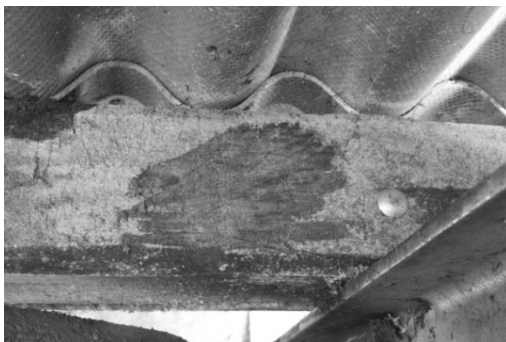
Figure 2. Wooden beams exposed to fungi.
