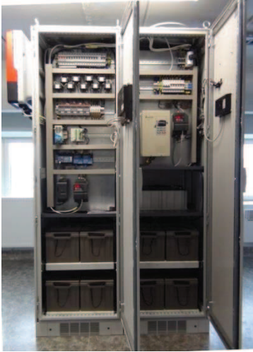
Figure 3. Laboratory main switchboard.
