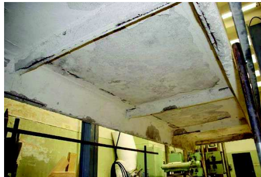
Figure 4. The condition of ribbed panel P8 before testing. Due to corrosion-affected spalled cover at the longitudinal ribs, ribbed panel P8 received grade 0 in the visual rating scale.
